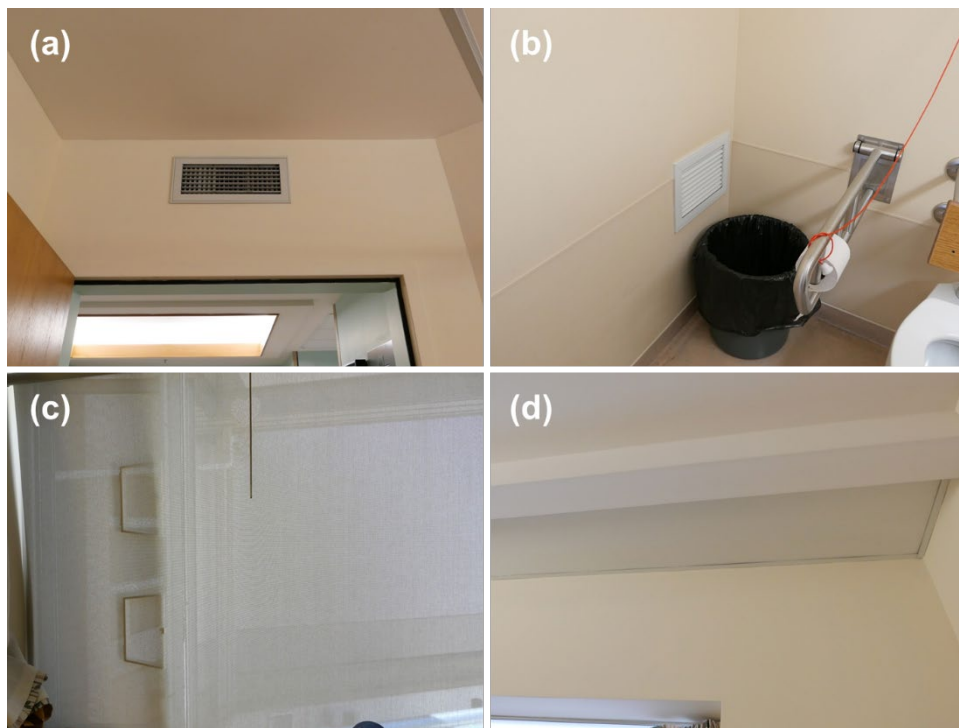
Figure 15. HVAC system terminal units for a typical resident room include (a) supply air diffuser above the door frame, (b) return air grille located in the washroom, (c) operable windows, (d) radiant ceiling panels above the window for perimeter heating.
