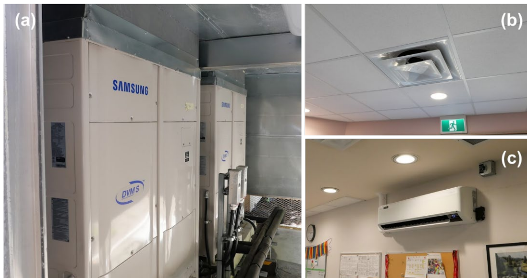
Figure 14. The heat pump system consists of (a) outdoor units, (b) indoor ceiling-mounted units serving the lounge areas, and (c) indoor wall-mounted units serving the Rehabilitation Service office.
