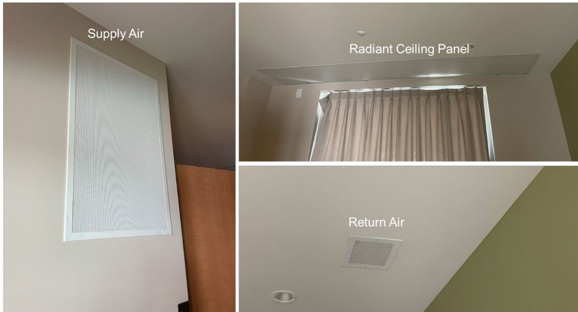
Figure 29. Ventilation terminal units in MHC patient rooms.
