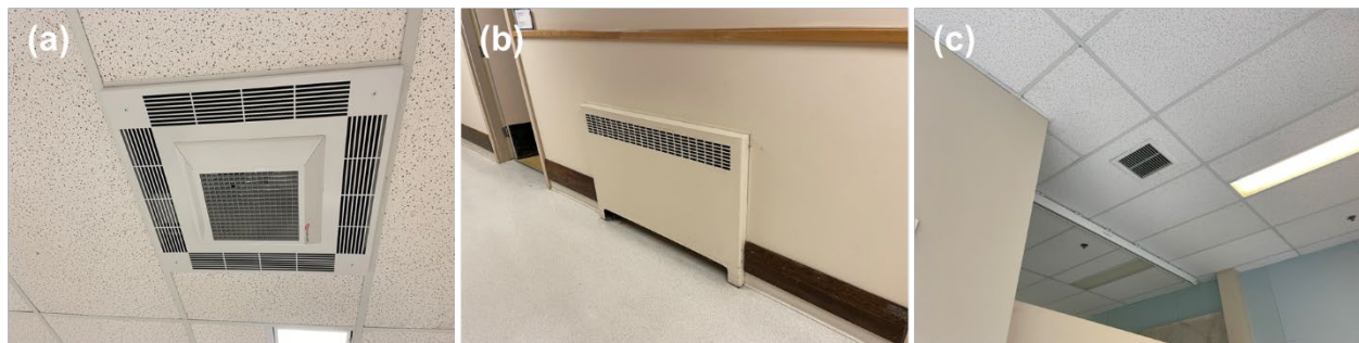
Figure 22. Heating units and exhaust fans in the Old Building include (a) ceiling fan heater, (b) perimeter radiant heater, and (c) ceiling exhaust fans.
